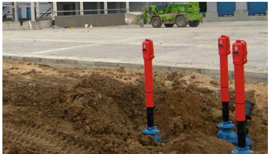
AVK series 34/00 post indicators for fire protection at FM Logistics, Petresti, Romania.
